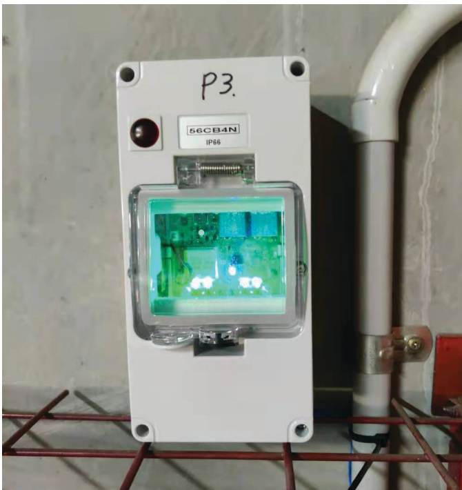
Installed Plexus Pump Sensor
